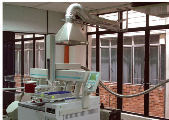
A flexible exhaust vent carries fumes outside.
