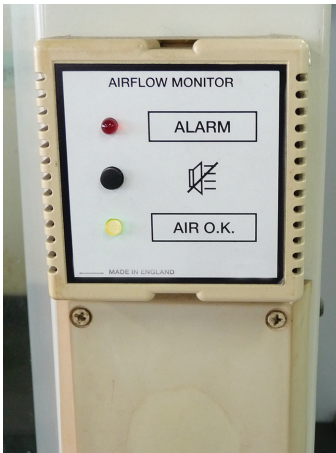
An air flow monitor sounds an alarm when exhaust air flow falls below a set level.
